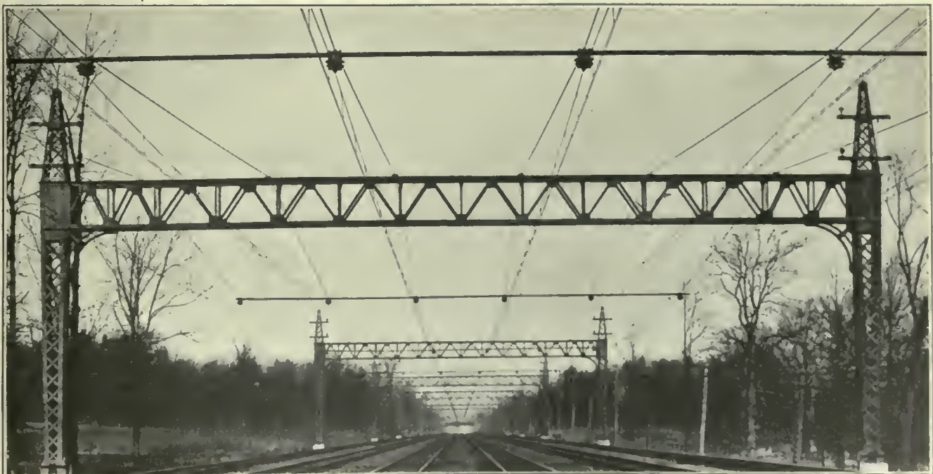
FIG. 516. OVERHEAD CONTACT SYSTEMS. Compound Catenary Overhead Contact System. 11,000-Volt Single-Phase Main Line Construction, New York, New Haven & Hartford Railroad, near New York City.
